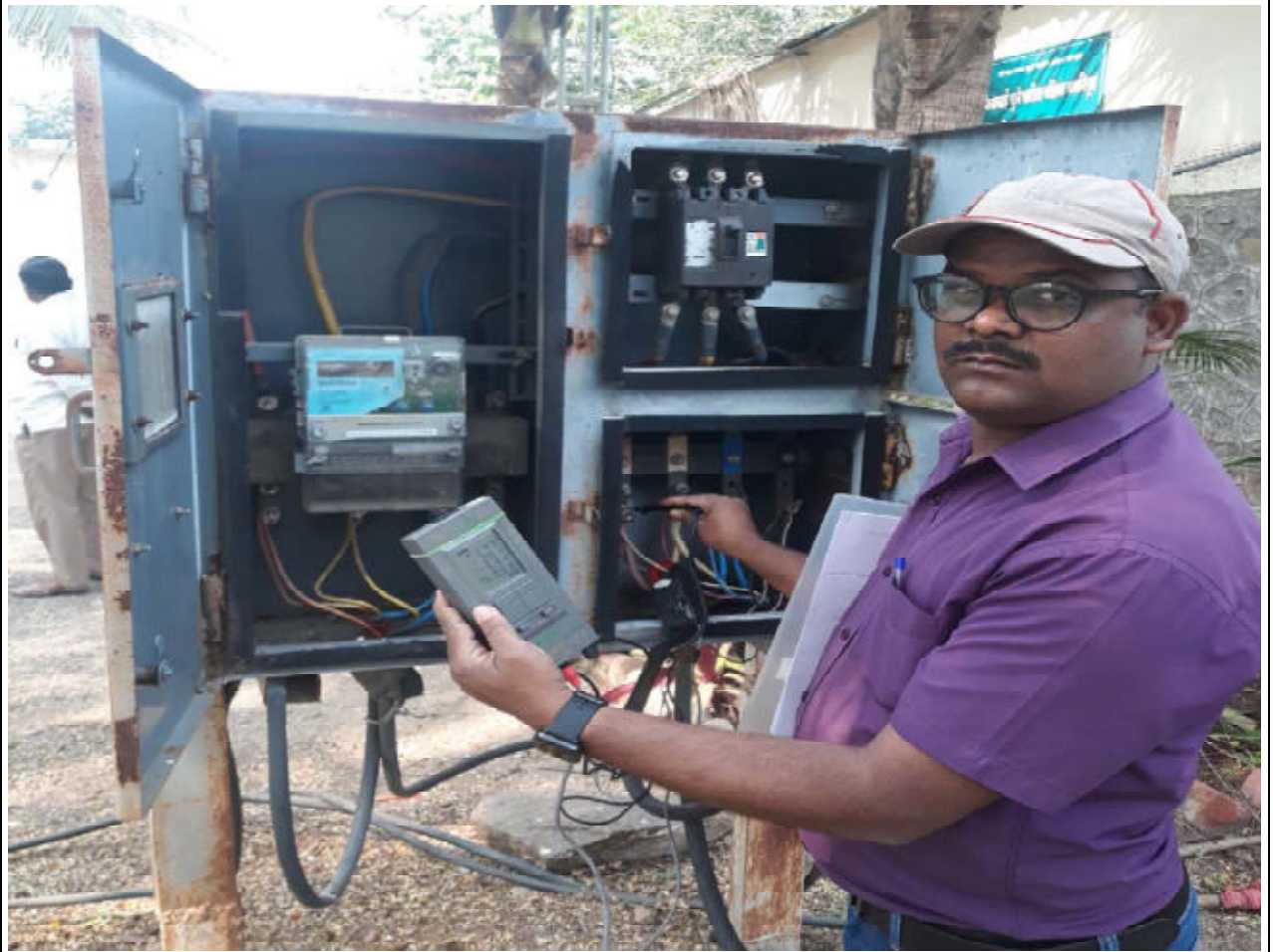
Load Measurement at Transformer and Hostel
