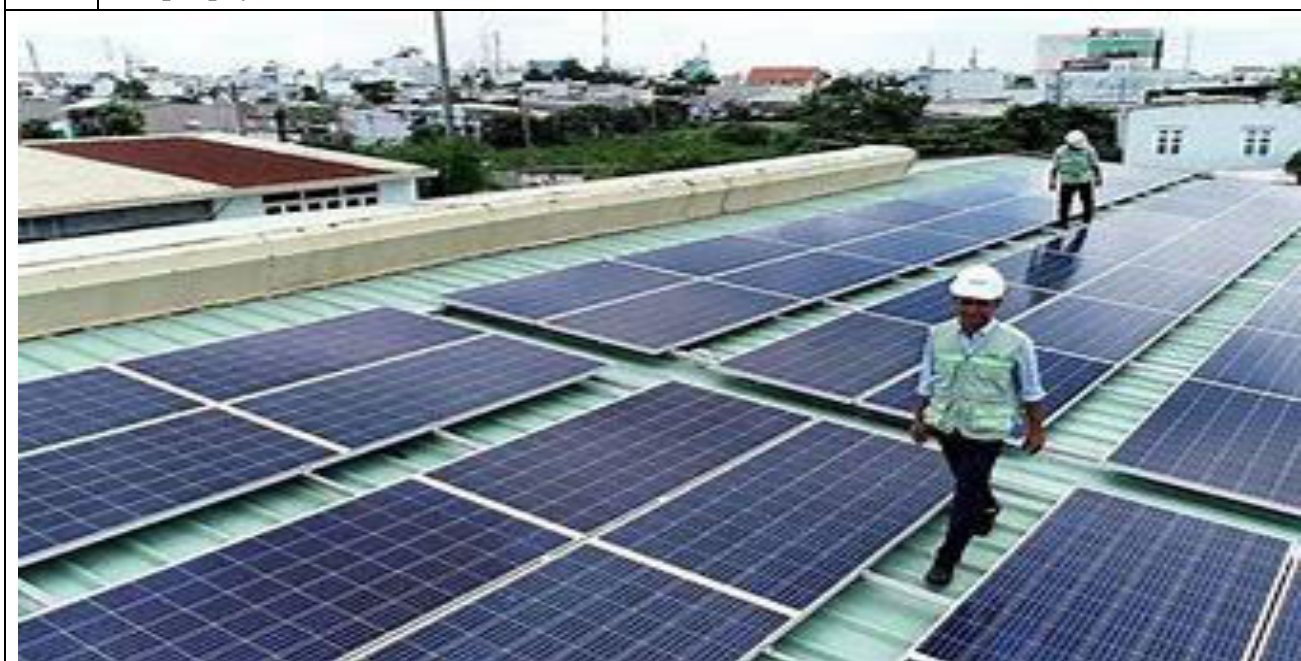
Figure 2 : Rooftop Solar Photovoltaic system
