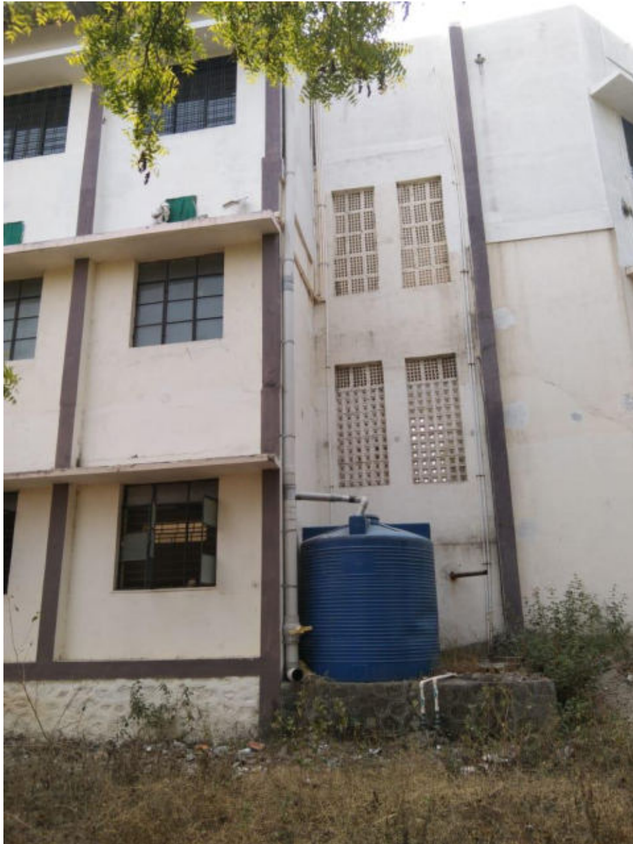
Rain water harvested at Tank
